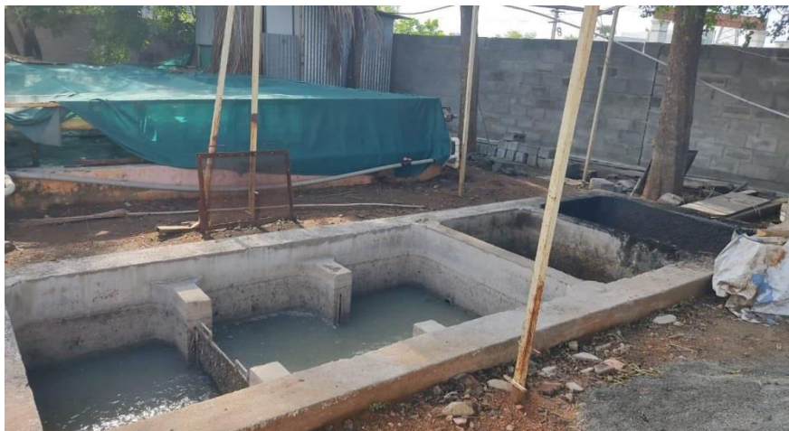
Fig.1 Food Waste Storage Tank
